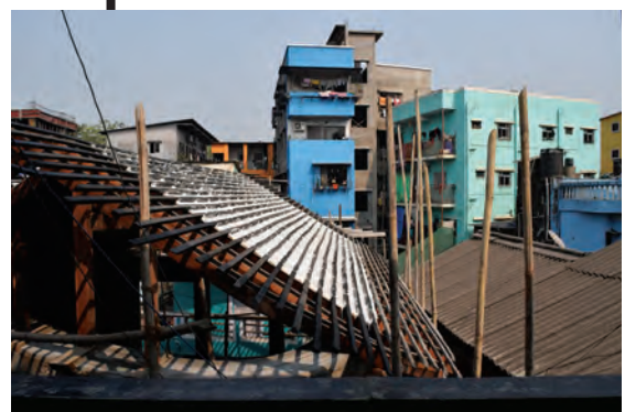
Artisan Abbas Galwani (top) is working with Urbz to revitalize a colonial building as a community hub, complete with a traditional pot tile roof.
