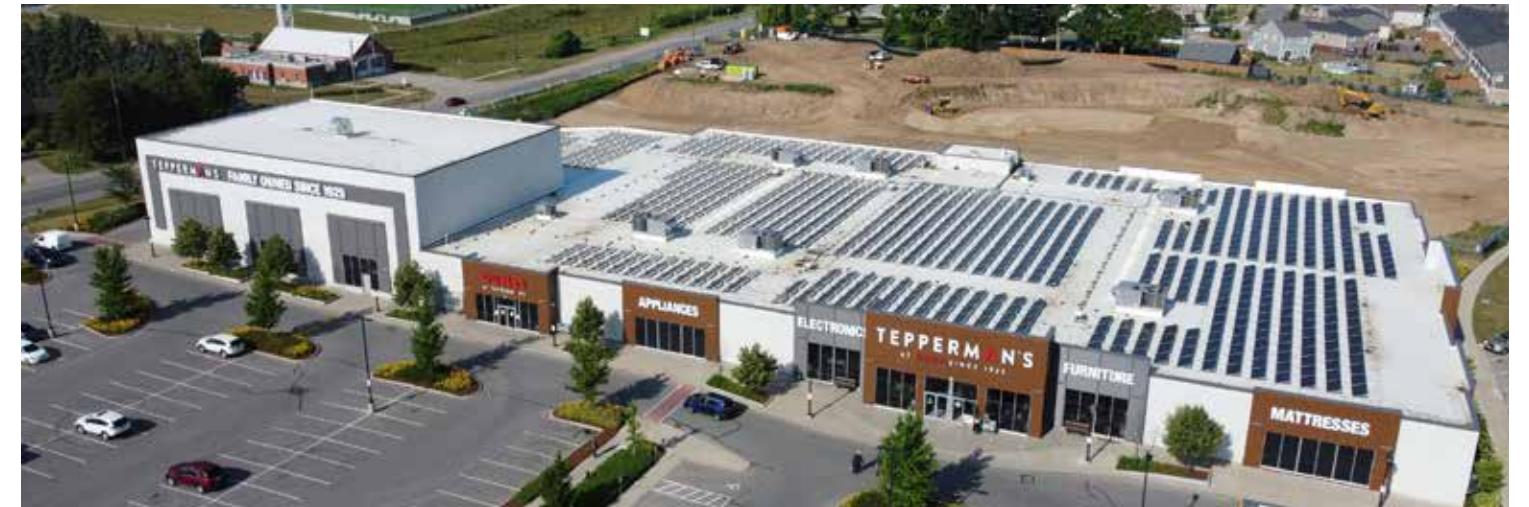
A sea of 914 solar panels covers the roof of Tepperman's Kitchener store. The solar array installation, designed as a ballasted system, was carried out by VCT Group.
